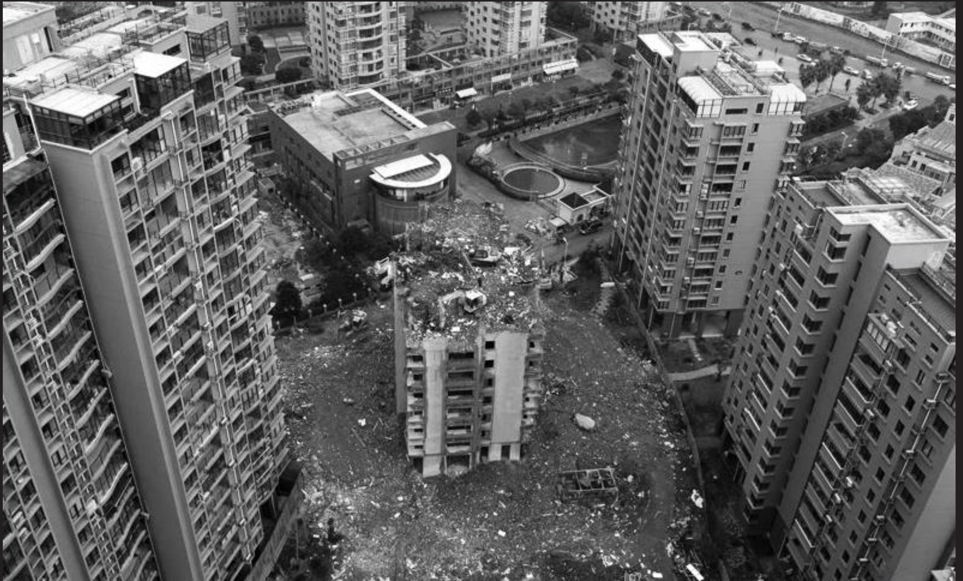
Residential buildings were demolished less than one year of completion, Taizhou, Zhejiang
